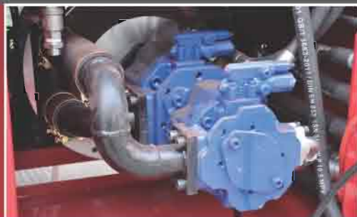
The Bosch Rexroth hydraulic oil pumps and motors, be driven by ABB electric motor. Supply the power to the rig.
